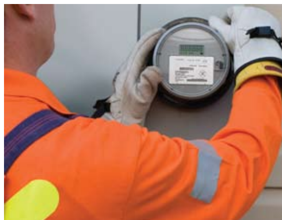
Smart meters will be installed in customer's homes starting in January 2009.
